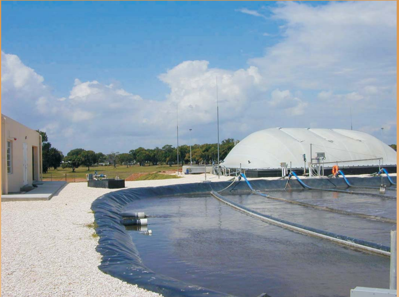
SKJÖLDGAS-plant for a brewery and beverage industrie with 0,2 million hl/a
